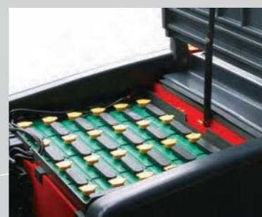
Full accessible 48 volt batteries with 400-600 Ah capacity are controlled by Danaher or Curtis AC control systems.
