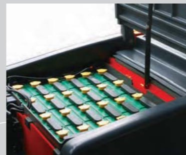
Full accessible 48 volt batteries with 400-600 Ah capacity are controlled by Danaher or Curtis AC control systems.
